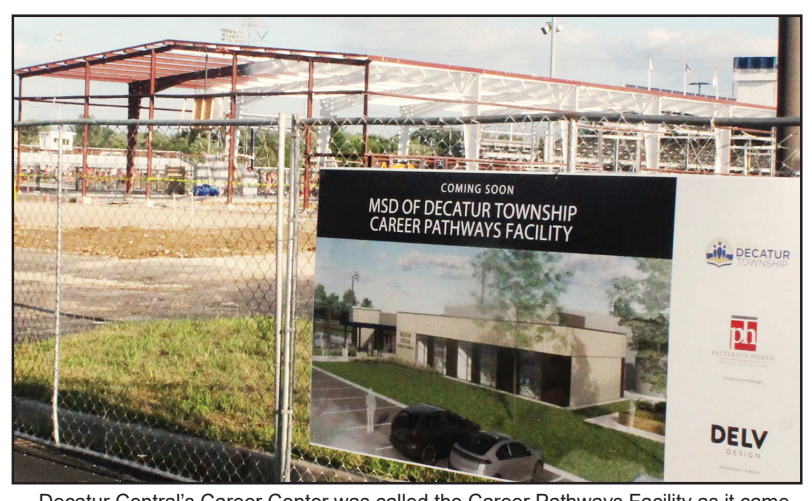
Decatur Central's Career Center was called the Career Pathways Facility as it came out of the ground last summer.
